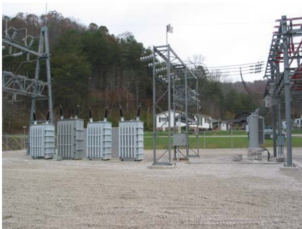
Transformer station near residential house before
