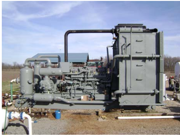
Natural Gas Compressor
