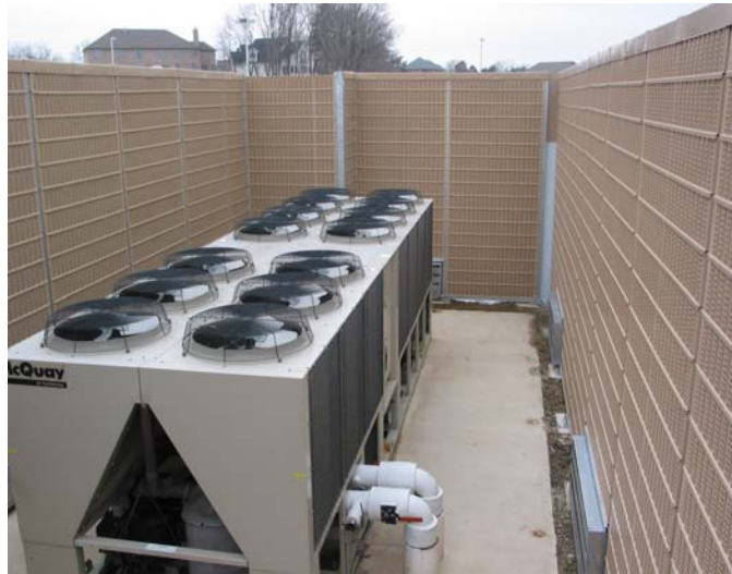
Sound Barrier Wall – McQuay Chiller
