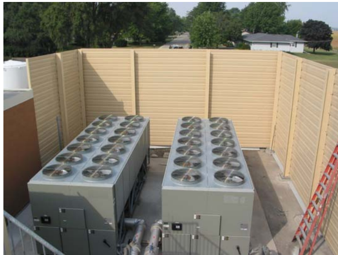
Sound Barrier Wall – two Trane Screw Chillers
