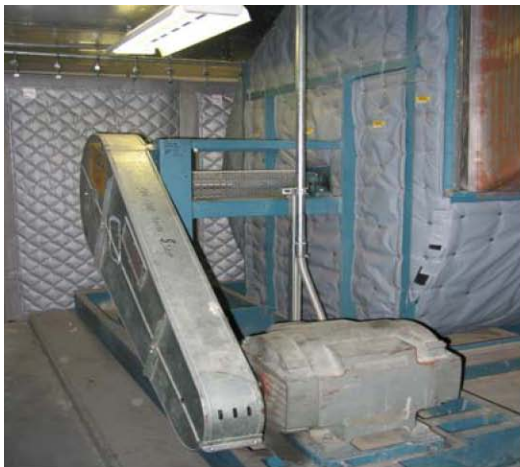
Blower casing shown with eNoise Control's removable sound blanket
