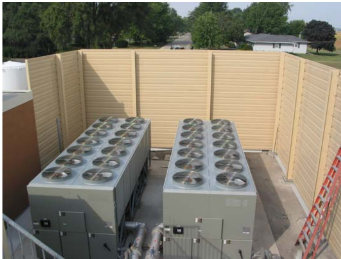
Sound Barrier Wall – two Trane Screw Chillers
