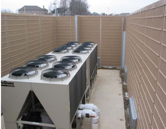
Sound Barrier Wall – McQuay Chiller
