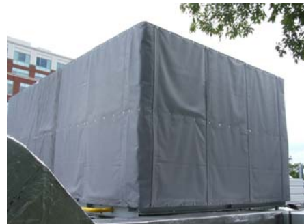
Outdoor blower after
